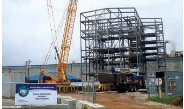
Pictured above, the Conyers, Ga. site is the first major boiler erection contract (of this type) PIC has worked on.
