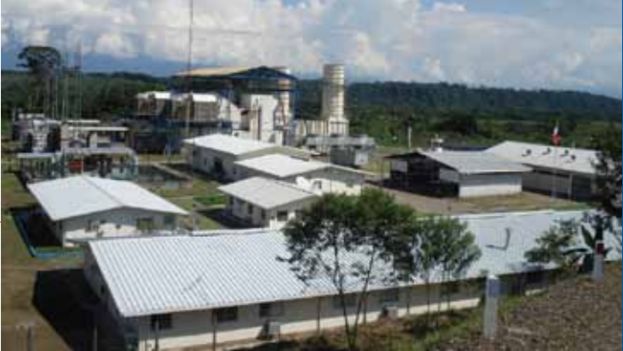
Aguaytia Power Plant - Peru
